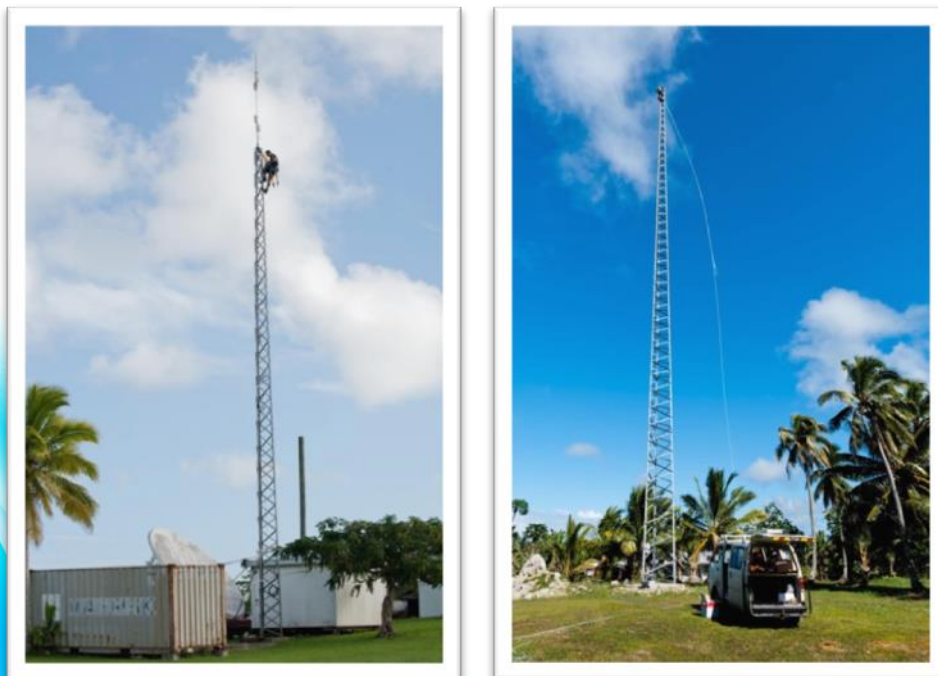
Wi-fi infrastructure maintenance by Rocket systems
