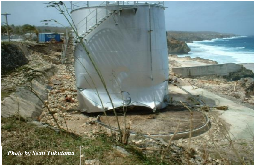
Fuel Depot in Alofi damaged by Tropical Cyclone Heta 2004
