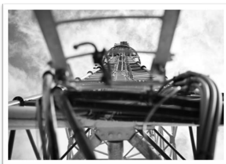
Communications infrastructure - Seikena tower
