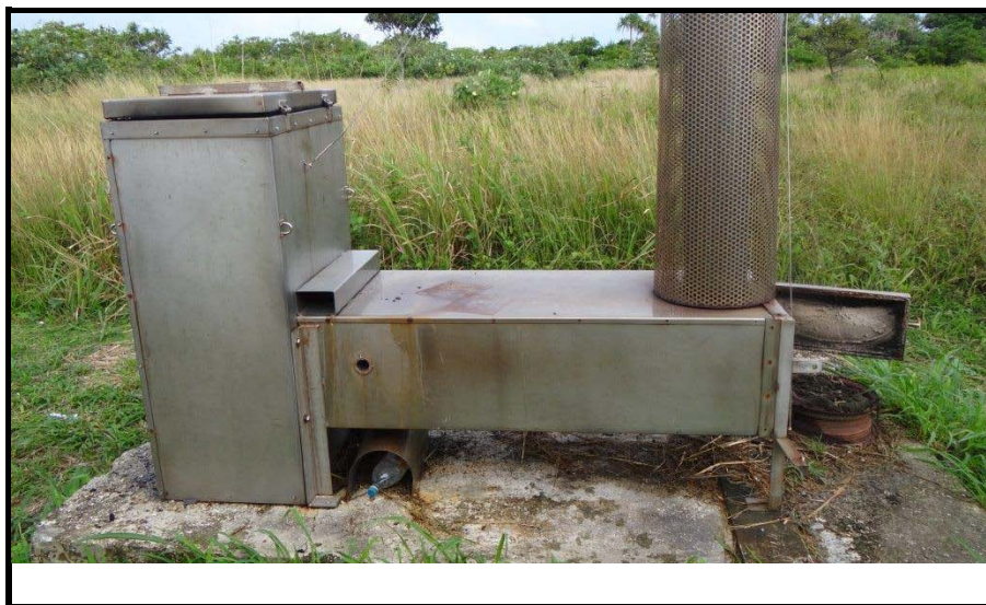
Photo 2: Wood fired incinerator, Niue Fooo Hospital, Niue (taken 20/05/2014 by Geoff Latimer ref:DSC04870)
